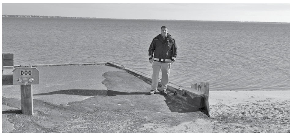
Brookhaven highway superintendent Daniel Losquadro recently inspected one of the more severely damaged road ends in Brookhaven Town, Moriches Island Road in East Moriches.
